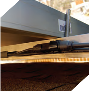
Cable Management in Rails
